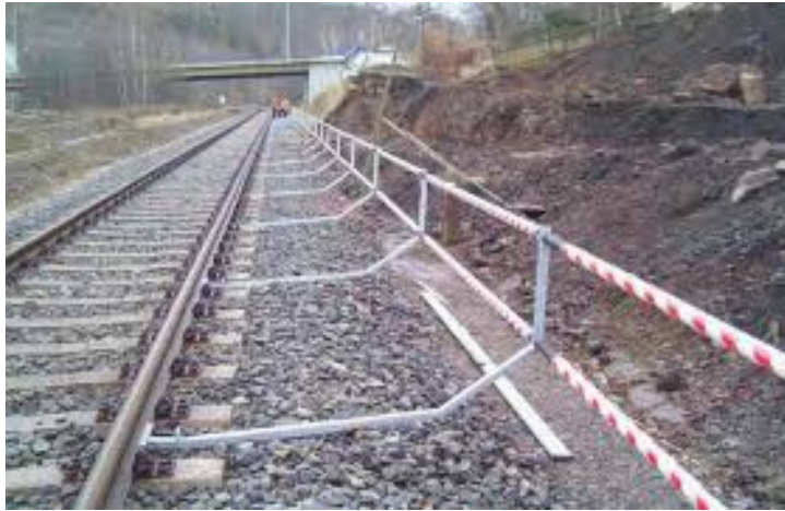
Figure 5 Safety Fences protecting a worksite from access to the Profile Gauge
