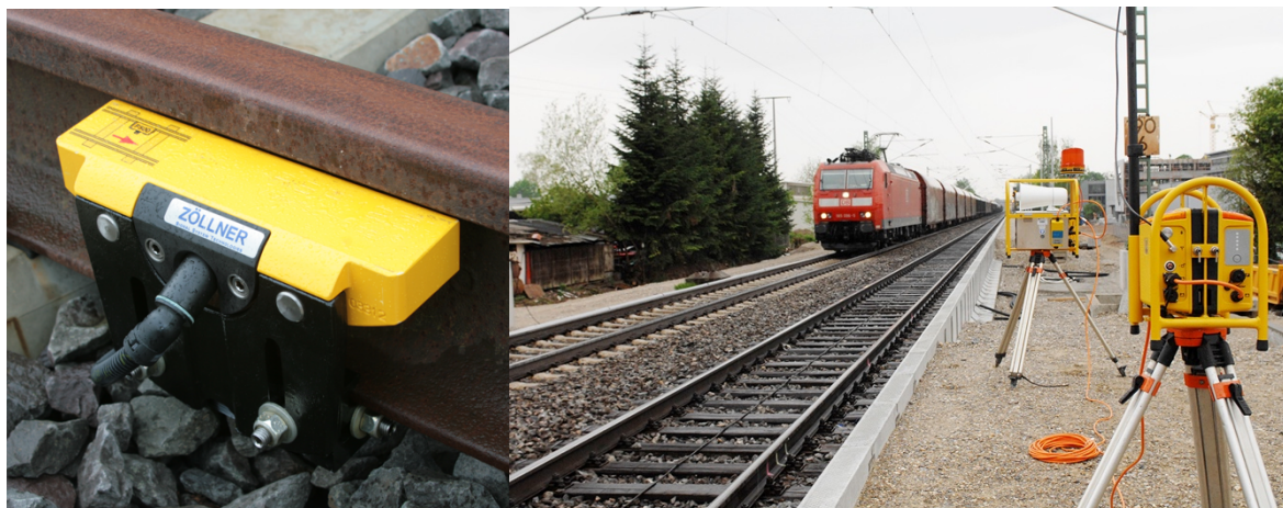
Figure 3 ATWS wheel sensor and trackside warning equipment (photos courtesy of ZÖLLNER).
